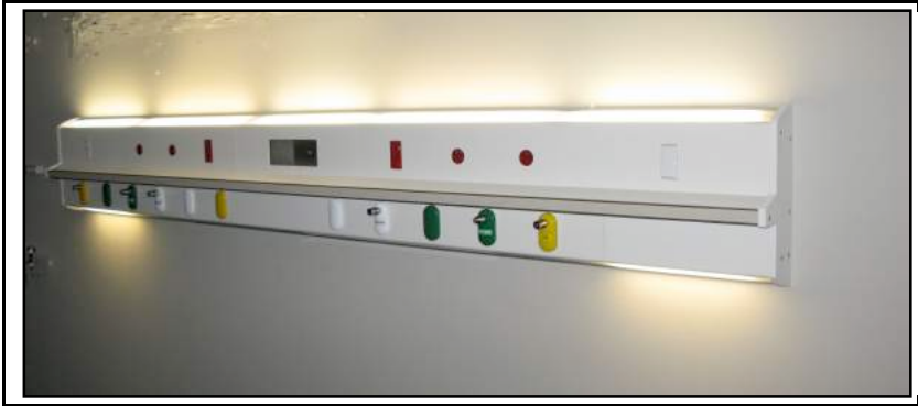
Fig 1 -1 Completely Installed MGR with lighting option
